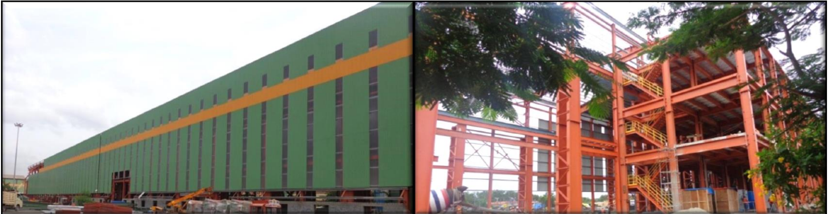
Electrical Steel Mill at Vijayanagar: expected to be commissioned by end FY15
